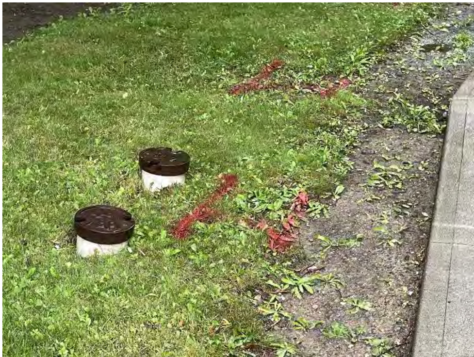
Photo 6: Two (2) water supply wells were observed at the Site east of the Site building at 165 Cross Avenue.
