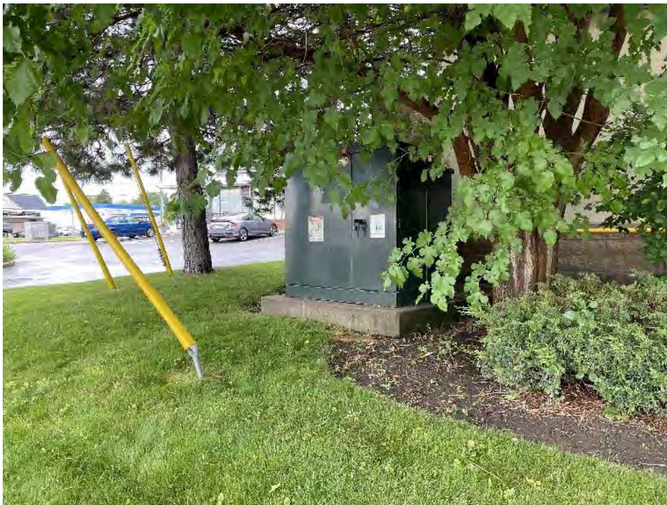
Photo 18: One (1) transformer was observed at the property located at 217 Cross Avenue, approximately 140 m northeast. Based on the label, it was manufactured in 2003, which is unlikely to contain PCBs.
