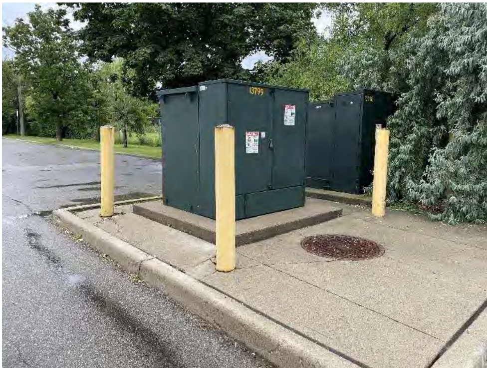
Photo 14: Two (2) transformers were located east of the building at 125 Cross Avenue, west adjacent, facing northeast. Based on the label, they were manufactured in 2017, which are unlikely to contain PCBs.
